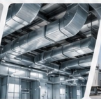
AIR HANDLING UNITS
