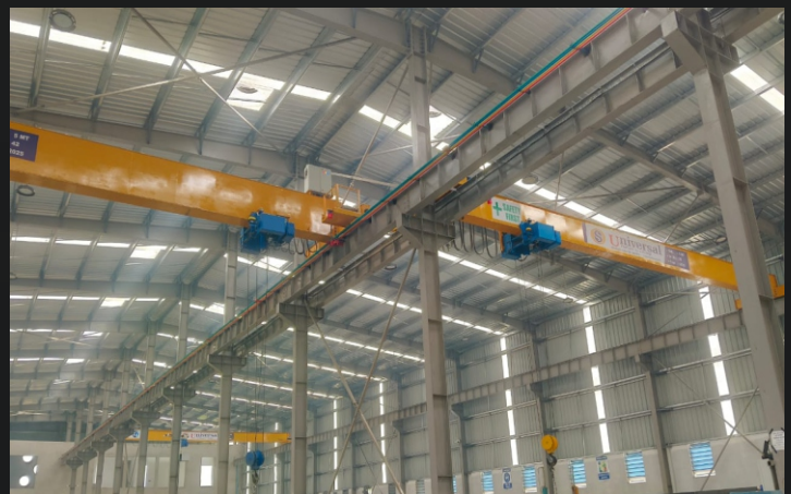
Multiple EOT Cranes
